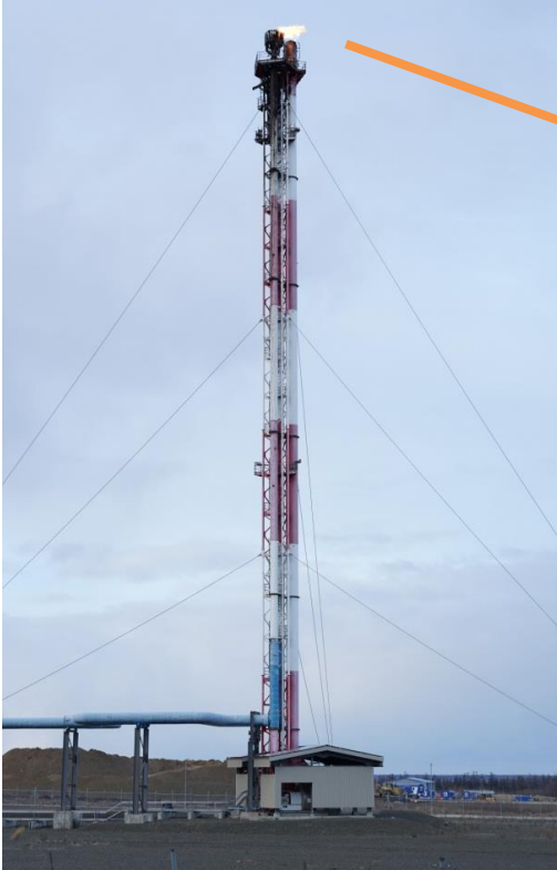
General view on Flare Stacks and Flare Tips. View from south.
